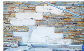
Delamination of Stone
