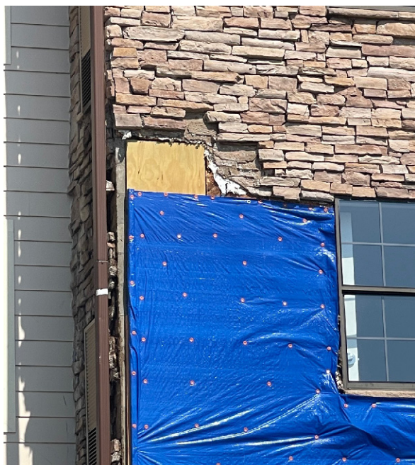
Traditional lath and scratch installations are vulnerable to moisture, leading to failures as seen above.
