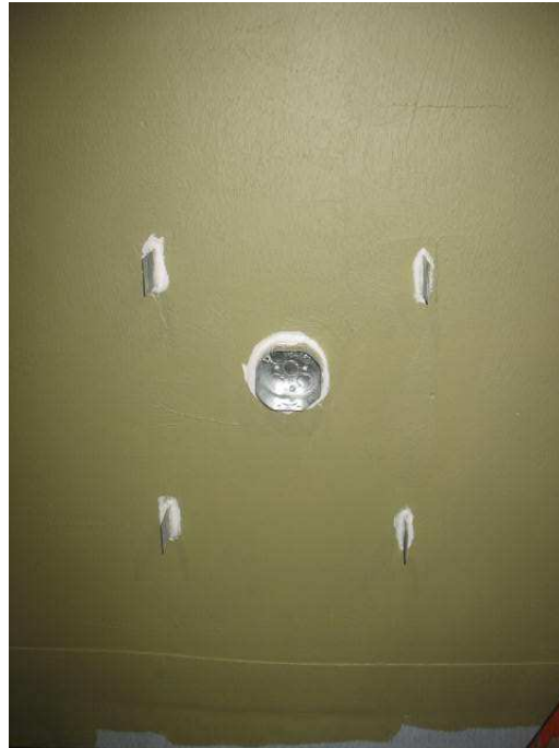
Figure E-11 – Application of MVIS Silicone Sealant around Brick Ties and Hexagonal Electrical Junction Box
