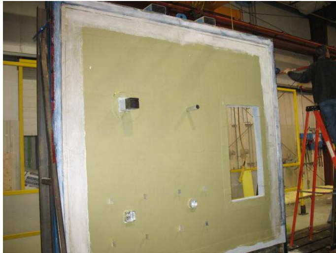
Figure E-9 – Application of LATICRETE Transition Tape Primer around Perimeter Wall / Specimen Transporter Frame Interface
