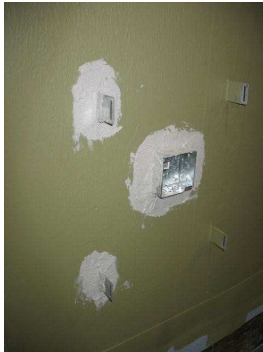
Figure E-10 – Application of LATAPOXY Waterproof Flashing Mortar around Brick Ties and Square Electrical Junction Box / Adjacent Brick Ties Sealed with LATICRETE Air & Water Barrier
