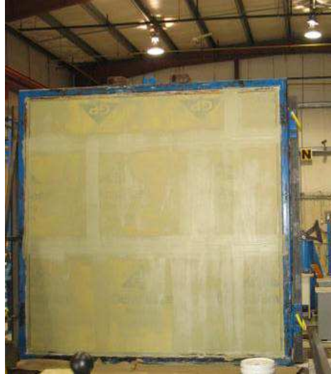
Figure D-1 – Sheathed Opaque Wall Section (Sheathing Joints Sealed and First Coat of LATICRETE Air & Water Barrier Applied)
